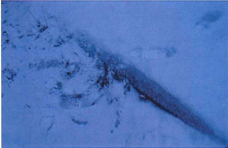
CK2285 Right fill settling
